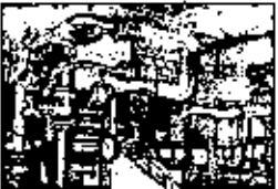
Fatty acid Spitting Plant High Pressure Pump
