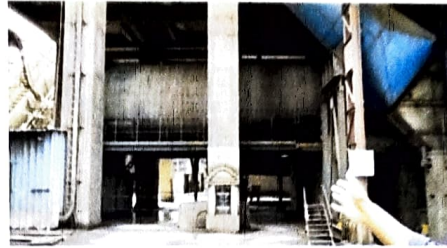
Proportioning equipment and finish Grinding mill
